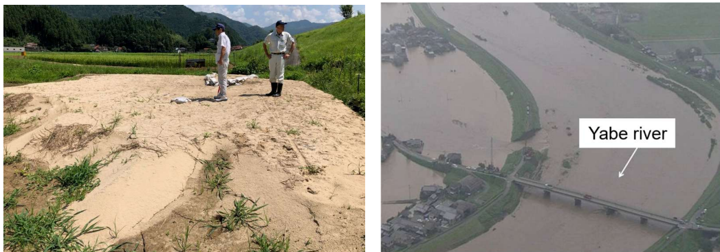
Figure 3.17 Left: Gono River levee sand boil in the Torrential rains in the western Japan of July 2018, Right: Yabe River levee breach by piping of July 2012 (MLIT)
