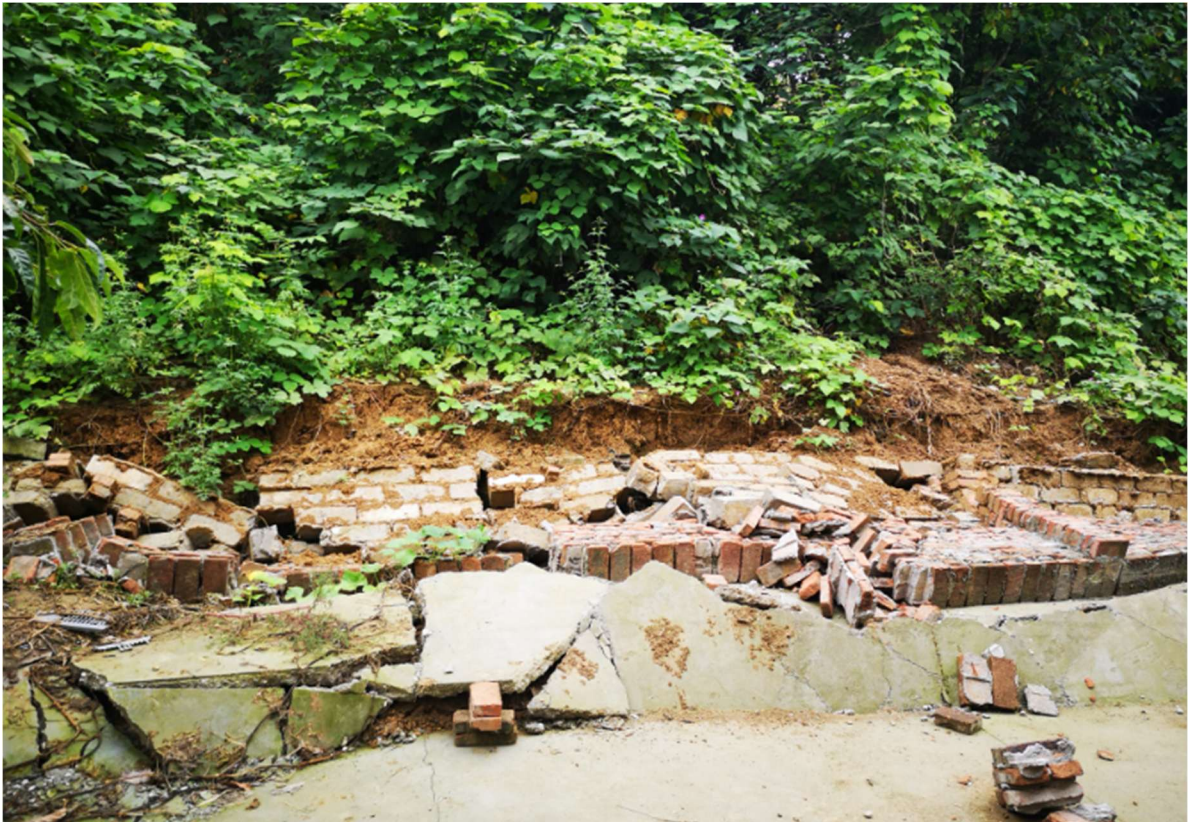
Figure 3.126 Landslide Leading Edge Bulge
