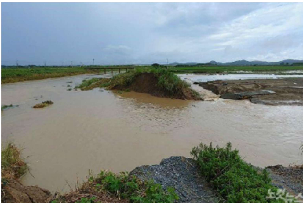
Figure 3.42 Levee failure along Munpyeongcheon, a tributary of the Yeongsan River. [5]
