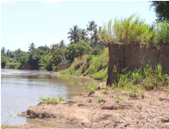
Figure 3.80 The condition of the remaining riverbank downstream de Intabo pumping station
