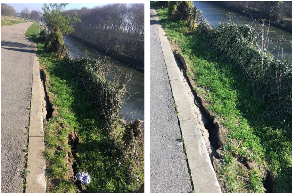
Figure 3.119 Pictures of subsidence and cracks near the roadway
