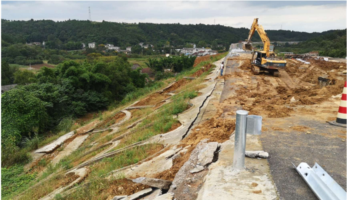
Figure 3.124 The Horseshoe-shaped Morphology of the Trailing Edge of an Embankment Landslide
