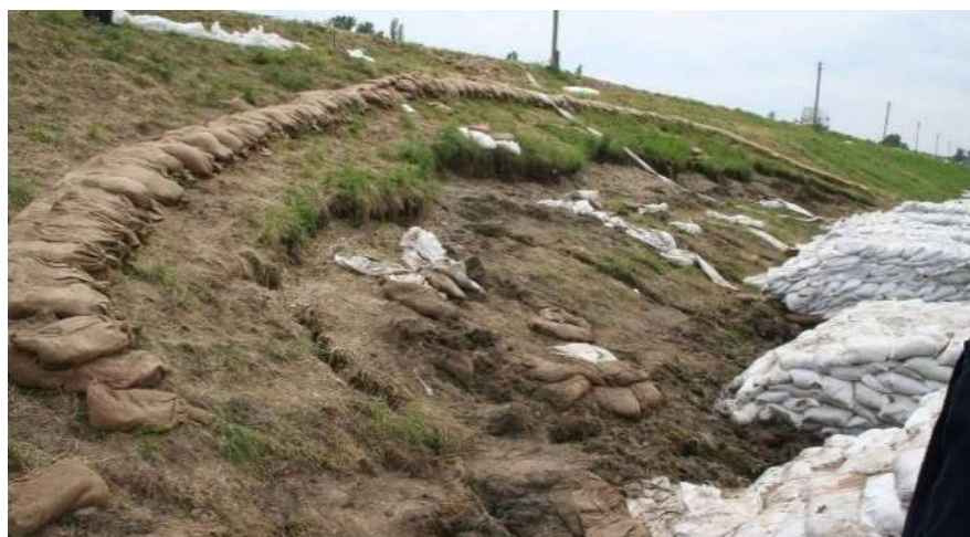
Figure 3.92 Slope sliding and temporary reinforcement
