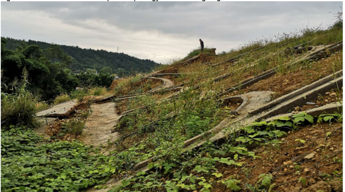
Figure 3.125 Landslides Protruding from the Embankment Area
