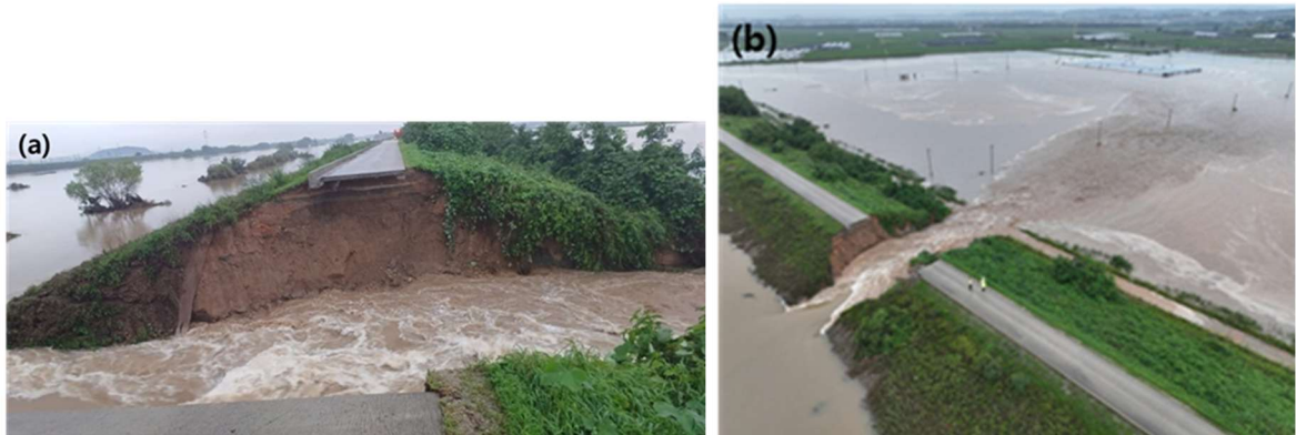
Figure 3.41 (a) Collapsed levee near Bridge Chungnam-si [3]; (b) Washed-out levee along the Geum River and Nonsancheon. [4]
