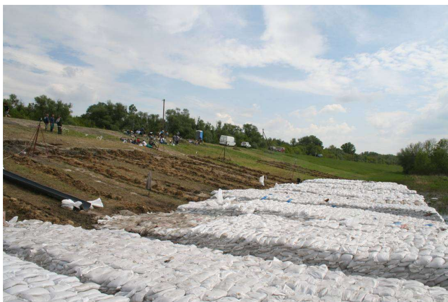
Figure 3.112 Slope sliding and temporary reinforcement
