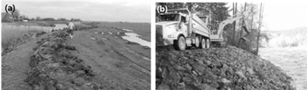
Figure 3.45 (a) Levee protected with a temporary floodwall system [8]; (b) Examples of Stone Masonry Construction Methods [8].
