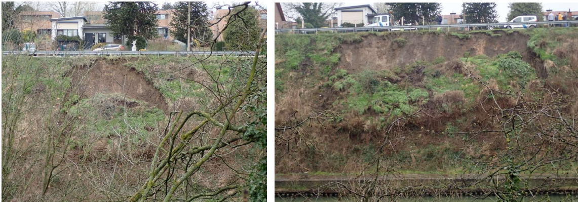
Figure 3.118 Pictures of the slope sliding.
