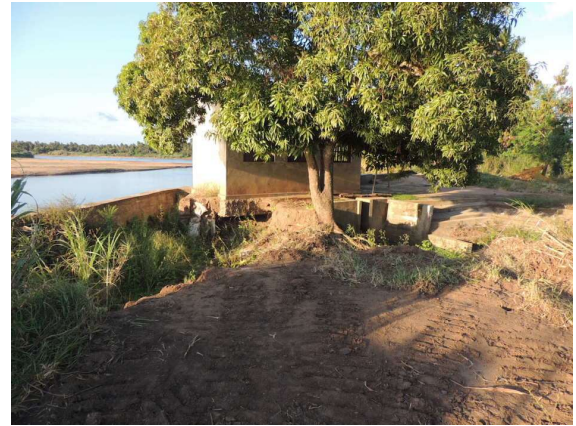
Figure 3.81 Erosion in the land side of the pumping station
